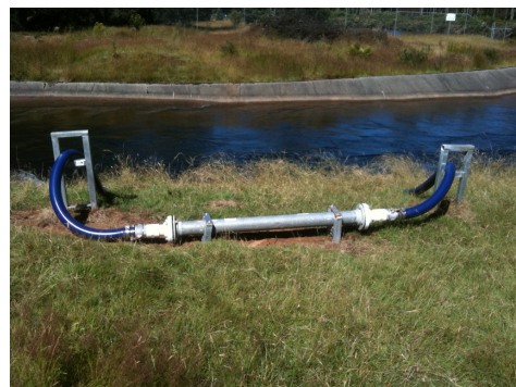
Fig. 3 Field pipe rig
